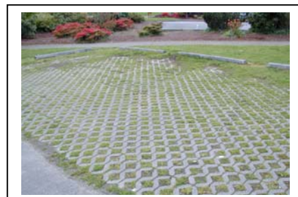
14. Permeable Pavers, Parking Lot
